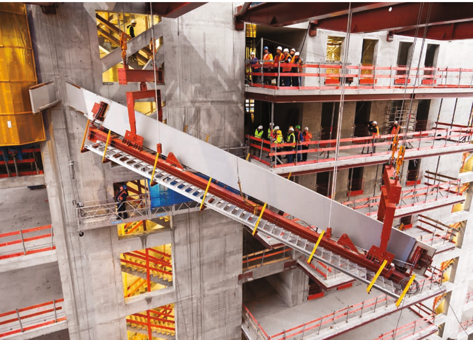
In November 2011 the first of a total of 14 trusses were mounted in the atrium between the two office towers. These trusses, together with the interchange platforms, serve to brace the two office towers.
