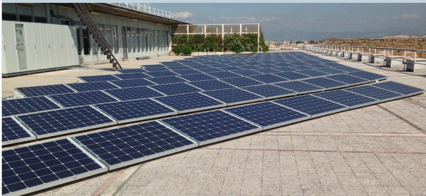
Photo 1: Solar energy panels installed at the Banknotes Directorate.
